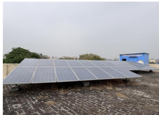
Image 43: Solar plates installed in GGSSS, Jacubpura
