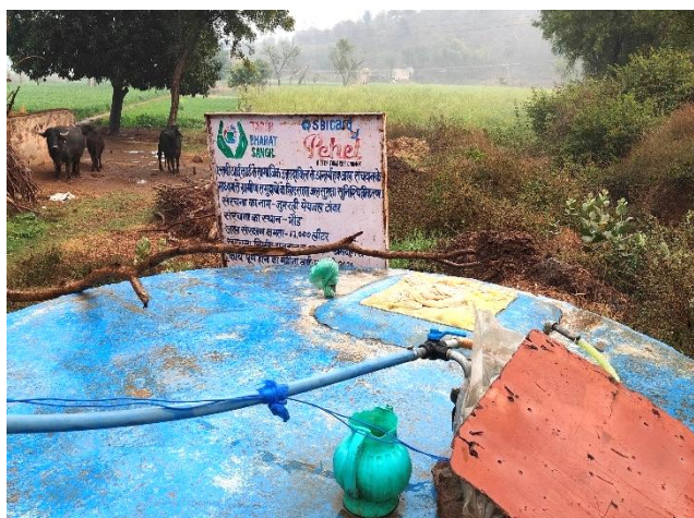
Image 65: Water tank with borewell connection at Basimeo village during field visit
