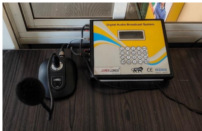
Image 31: Public announcement system installed under the project
