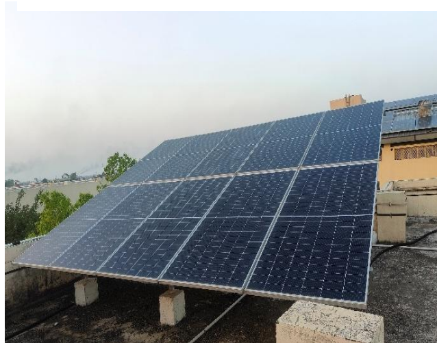
Image 30: Solar panels installed on the school terrace under the project.
