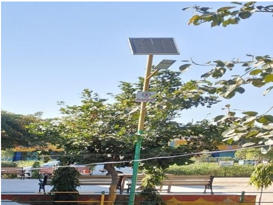
Image 6: One of the many solar streetlights installed in the Badagaon village
