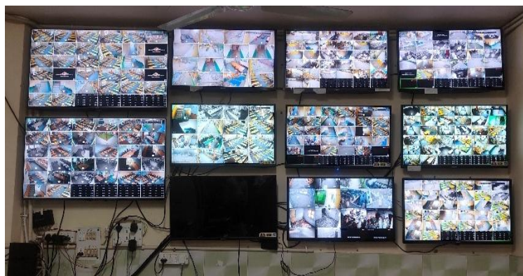
Image 32: Upgraded Surveillance Room with Additional Monitoring Screens and CCTV Camera Feed
